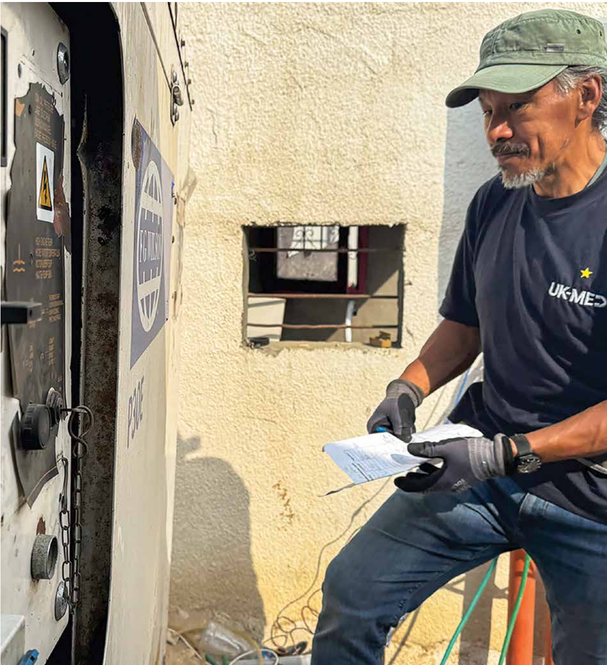
OSL staff conducting a maintenance check on a generator, Gaza, Occupied Palestinian Territory, 2024. © UK-Med
